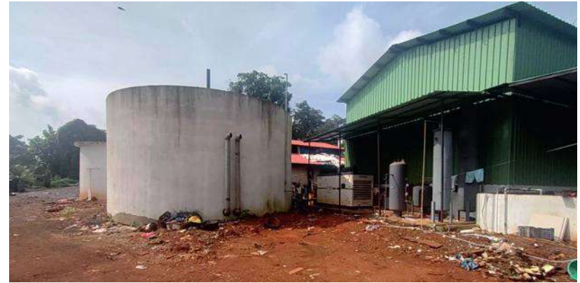
5 TPD Biogas Plant at Penha De Franca
